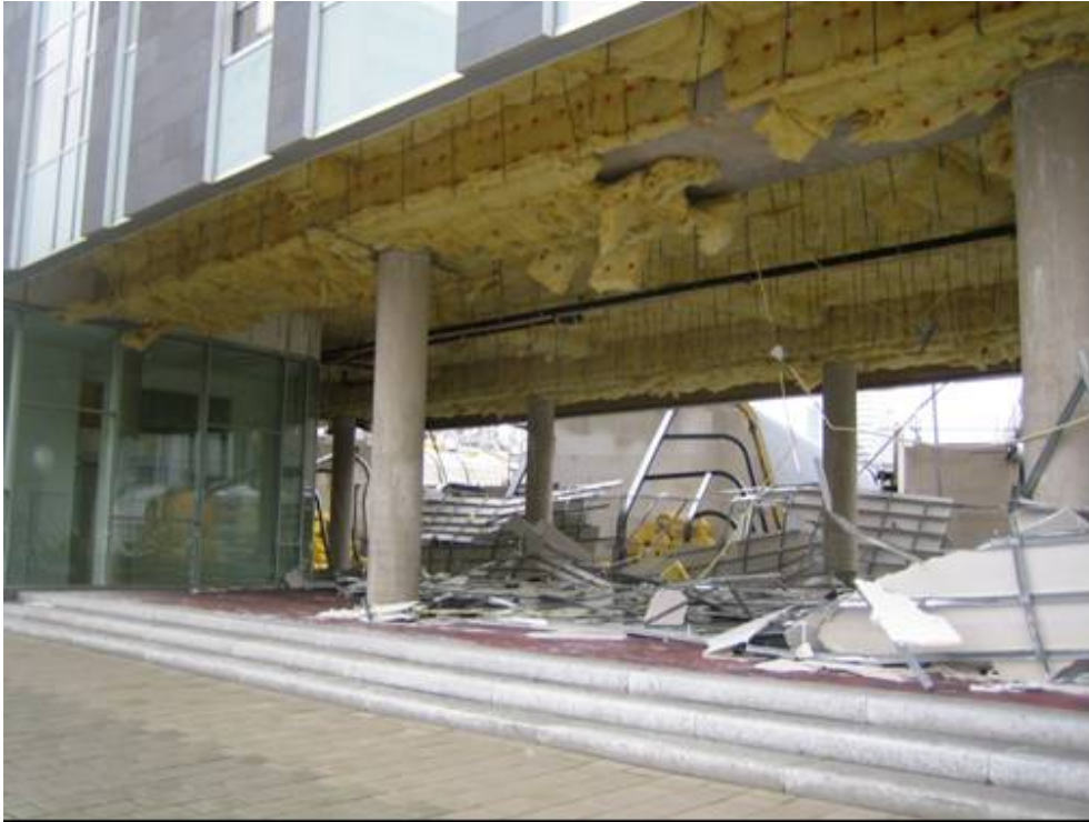
(Insured) storm damage to an outside ceiling: A situation not covered in standard building codes
