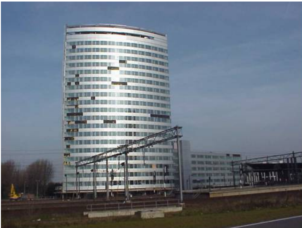
Storm damage to a light weight façade (wind was coming from the left)
